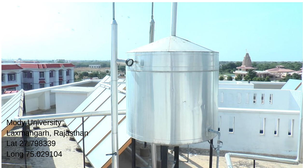
Use of Solar Water Heater in hostels Building
